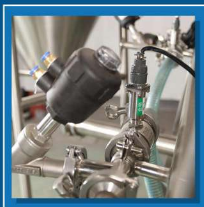
Flow Meter to Control Liquid Adding
